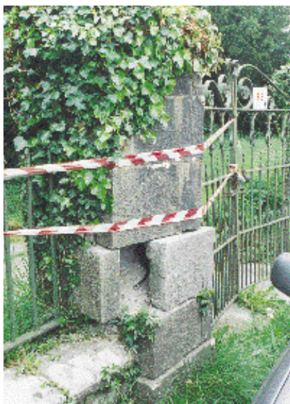
Entrance pier in need of repair, showing relative thinness of stones
